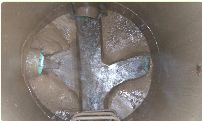
What should be flowing into this sanitary manhole on Railway Ave is sewage. But this photo shows that during periods of high inflow and infiltration (when this picture was taken) what is actually flowing into the system is a lot of relatively clean water from run off and sump pumps.
